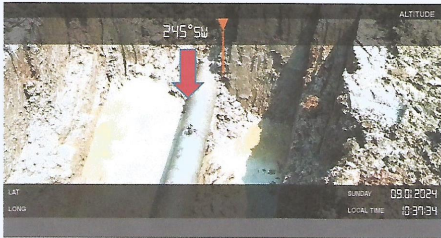
Pic1: Showing one (1no.) 2" nipple illegally installed on the pipeline
